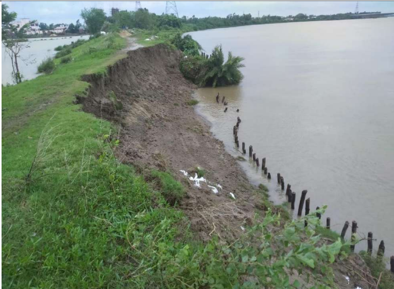
Damage of Keradagada Altnaga saline Embankment on Hansua right due to Cyclone "YAAS"
