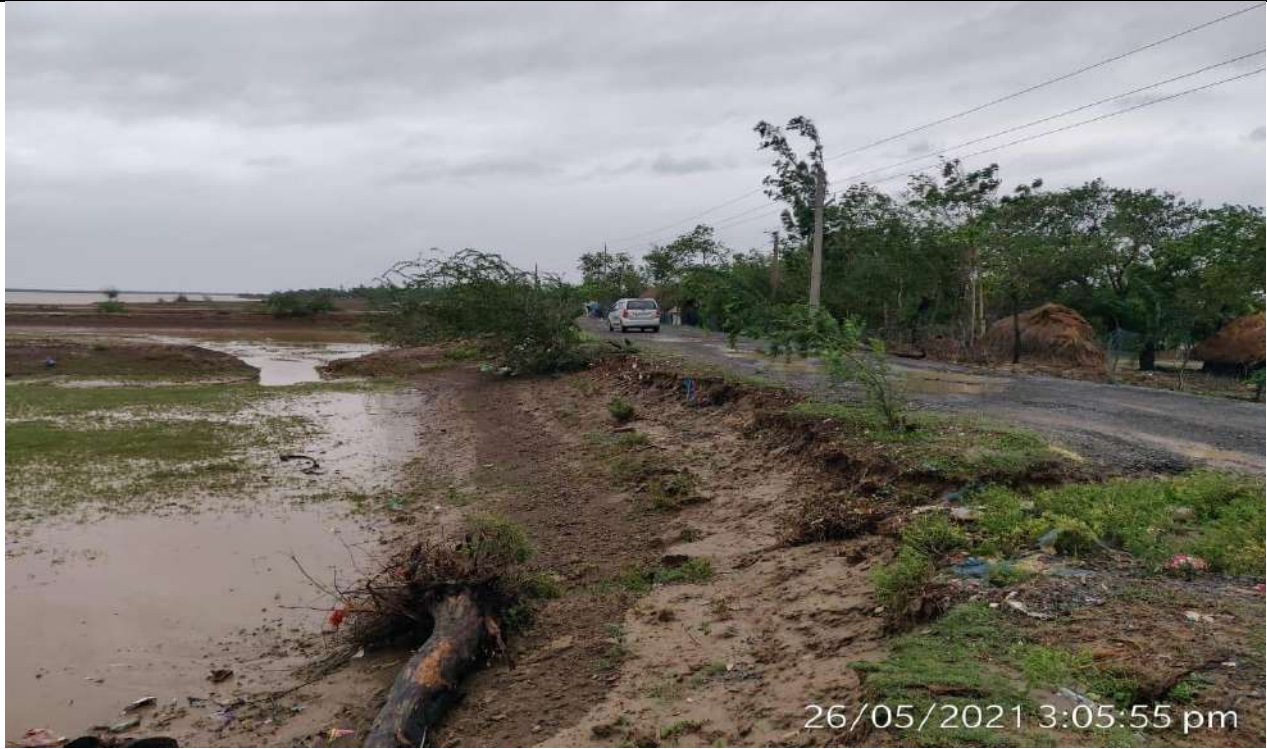
Damage of Naliatapatia Talachua Saline Embankment due to "YAAS"
