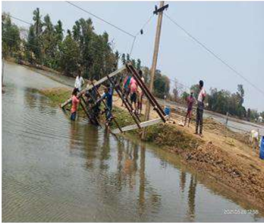
Broken DP Structure
