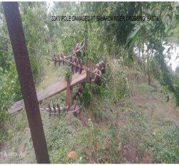
33 kV Pole Damage
